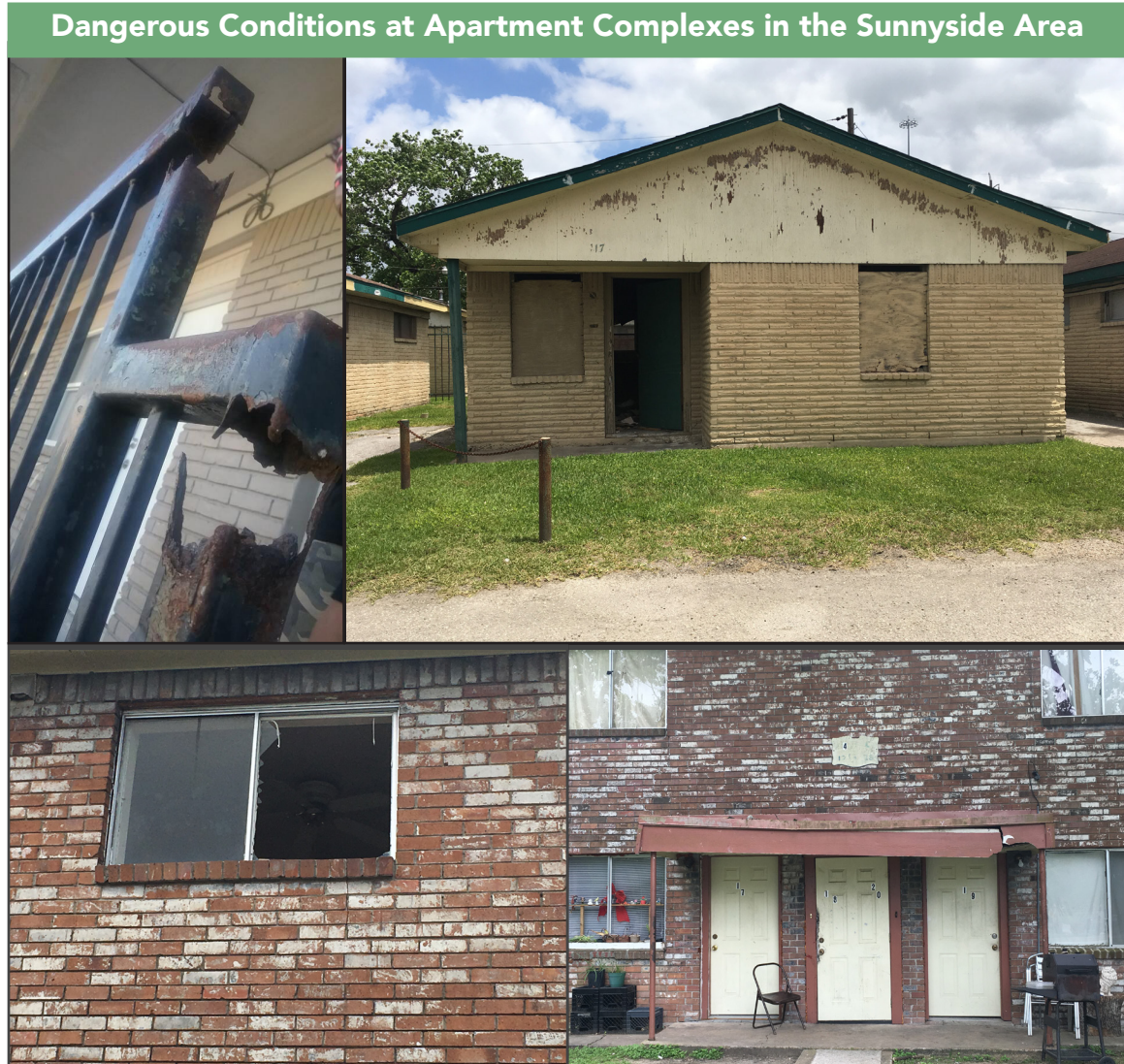
From top left clockwise: balcony railing at Jarmese Apartments, unsecured unit at Tierwester Village, sagging front porch roof at Belfort Townhomes, and missing second-story window pane at Belfort Townhomes
